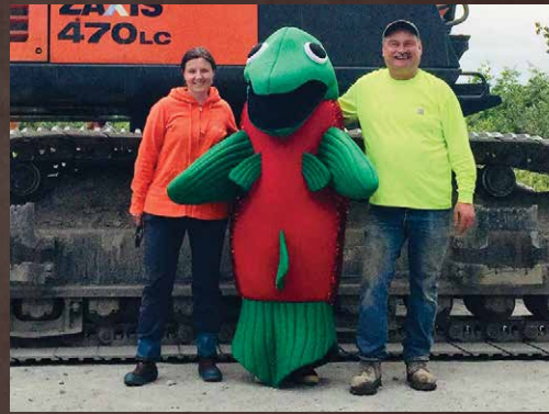
Lisa Docken and John Baenon (Wilson Construction) with Ruby the sockeye salmon celebrating the last of three culverts being placed on the Copper River Highway this summer! Photo by Amanda Williams
