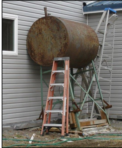
The set up of this tank makes it very vulnerable to damage from an earthquake or a flood.
