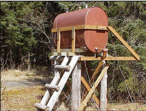
Check for tank stability. Legs for tanks should be resting upon a solid foundation. The bottom of the tank should be off the ground and clear of debris.
