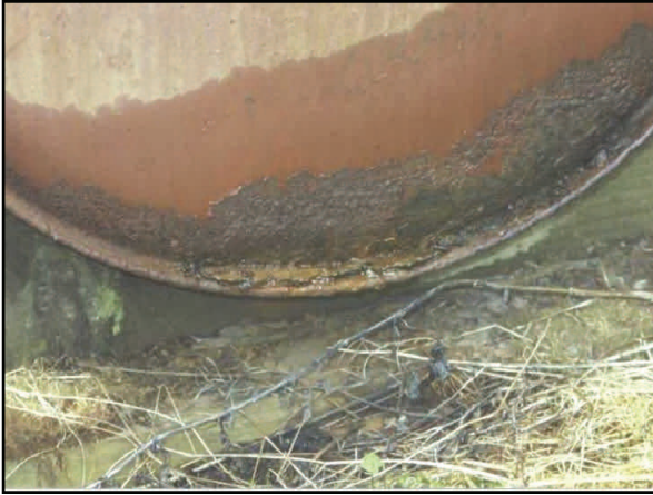
Replace your tank if it is rusting or if the tank appears damp! Painting tanks with a rust inhibitor paint will prolong the life of your tank.
