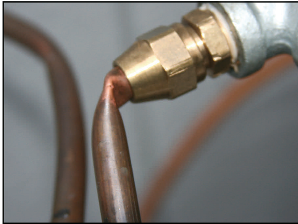
Check fuel lines to make sure they are not damaged or leaking. Pay close attention to connections or joints which can fail.
