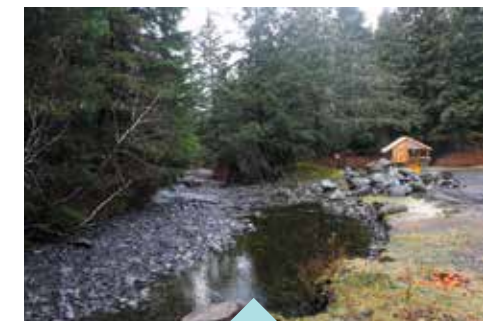
Bank erosion before restoration.
